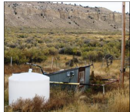
Domestic water well and stock water tank for pipeline.
